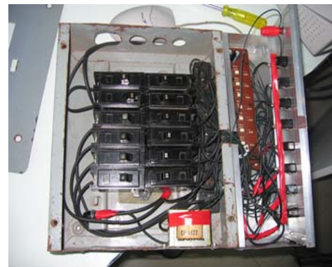
Figure 12 : The Panel Board Breaker and the Interface
