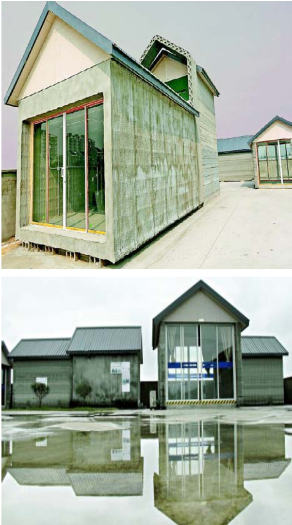
Figure 1 : Houses built by Shanghai WinSun Decoration Design Engineering Co., Ltd. within one day by using the technology of 3D printing(Photos:Liangfeng)
