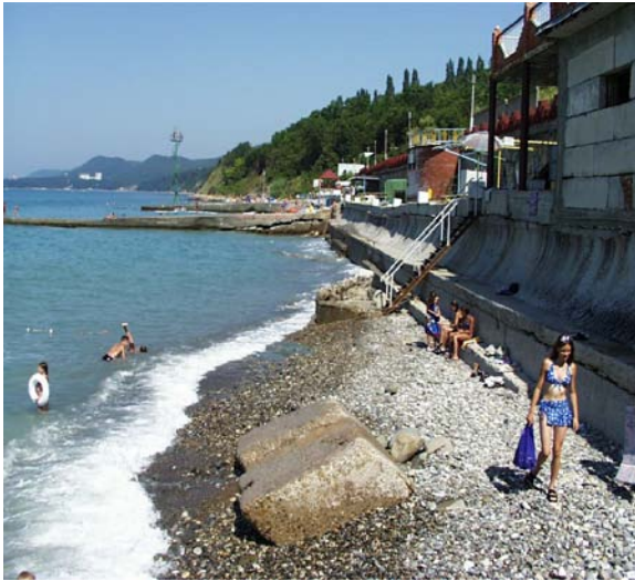
Fig. 12: Example of destruction of a wave protective wall. The beach near the wall is small
