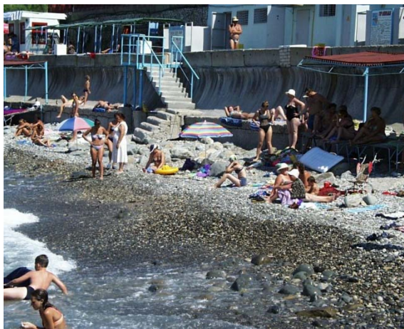
Fig. 13: Example of destruction of a wave protective wall. The beach near the wall is small
