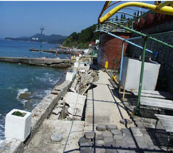
Fig. 11: Destroying of the wave-breaking wall from the marine and coastal party for want of a wave
