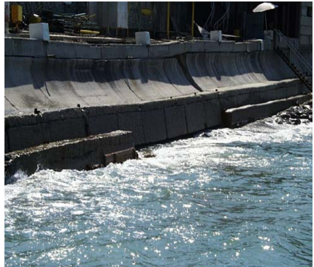
Fig. 9: Destroying of the wave-breaking wall from the marine and coastal party for want of a wave
