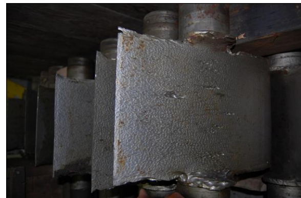
(a) Eroded guide vanes
