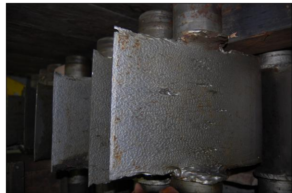
(a) Eroded guide vanes
