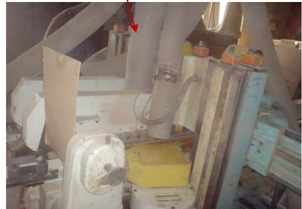
Figure 3 : Photographic view of conventional dust collection system
