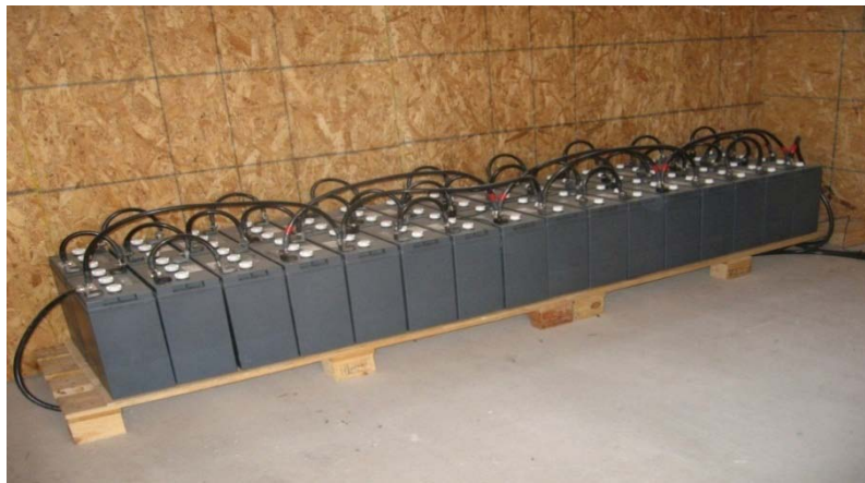
Figure 7 : Practical battery bank [13]
