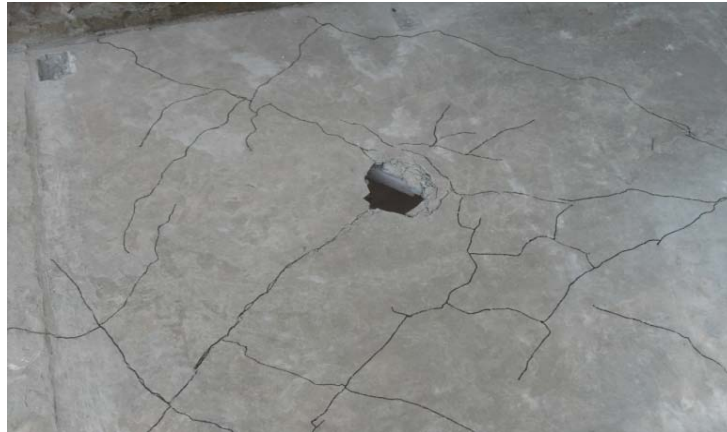
Figure 15 : Crack at Point d
