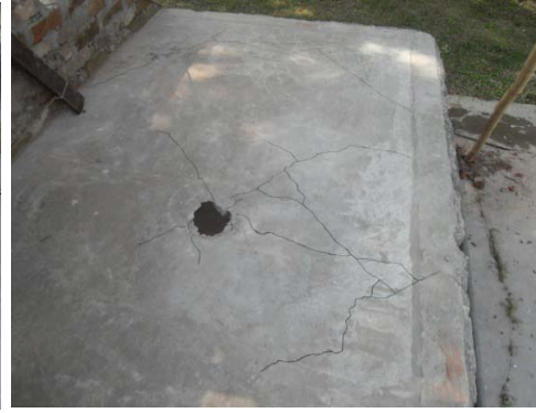
Figure 14 : Crack at Point e
