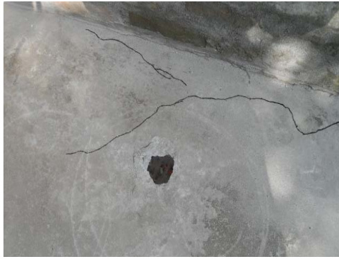
Figure 13 : Crack at Point c
