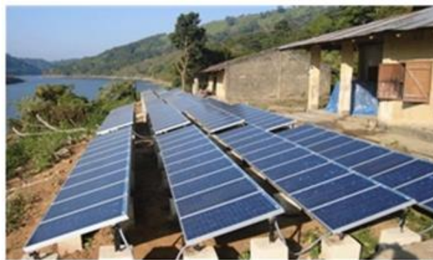
Figure 6 : Solar panels at Rangamati
