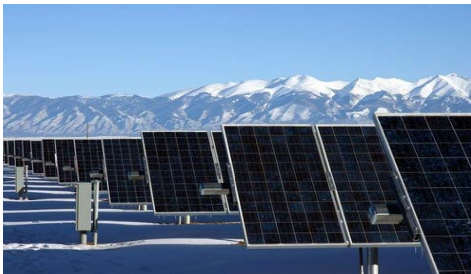
Figure 14 : Seasonally adjusted fixed-axis photovoltaic panels at the Sun Edison photovoltaic power plant near Alamosa, Colorado
