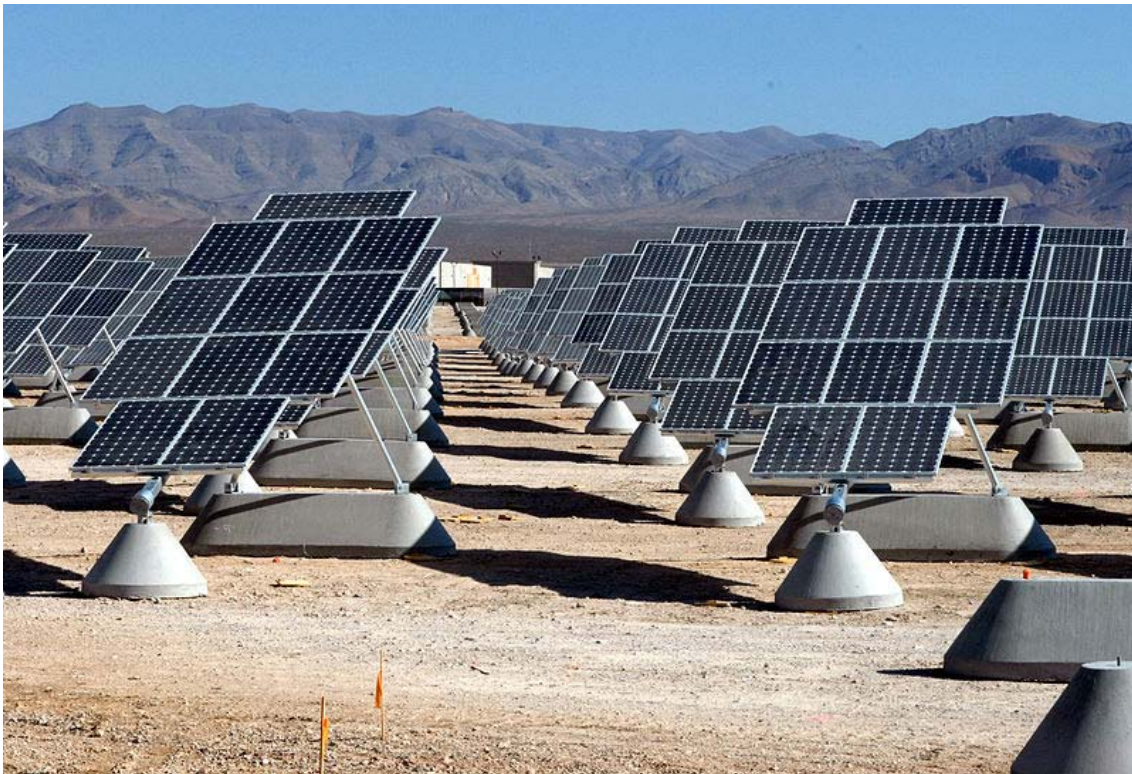
Figure 17 : Single axis trackers with roughly 20 degree tilt at Nellis Air Force Base in Nevada, USA. The arrays form part of the Nellis Solar Power Plant. Credit: U.S. Air Force photo by Senior Airman Larry E. Reid Jr,
