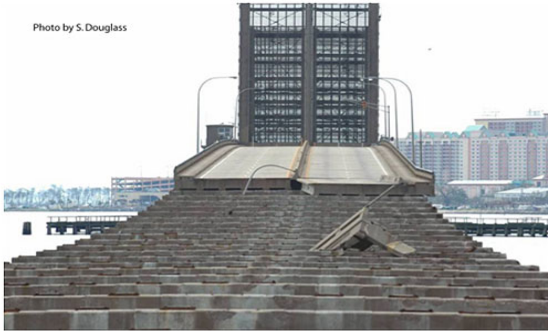
Figure 5 : US 90 bridge over Biloxi Bay, Mississippi was damaged by Katrina. Since the spans at higher elevations were not removed, the wave setup on top of the storm surge is more important than the wind loading (photo looking southwest from Ocean Springs 2/19/06, from FHWA-NHI-07-096)
