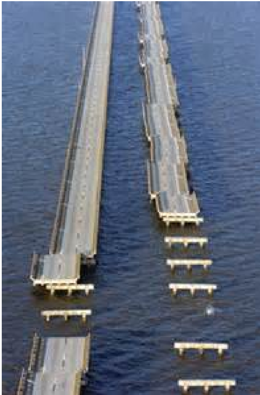
Figure 4 : Interstate I-10 over Mobile Bay damaged by Hurricane Ivan in 2004 (From FHWA-NHI-07-096). According to FHWA, the wave setup on top of the storm surge was the cause
