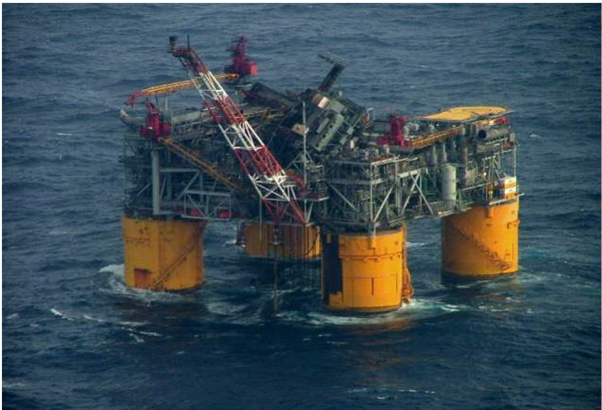
Figure 3 : Mars platform showing damage from Hurricane Katrina in 2005 (From http://en.wikipedia.org/wiki/Mars_(oil_platform) )
