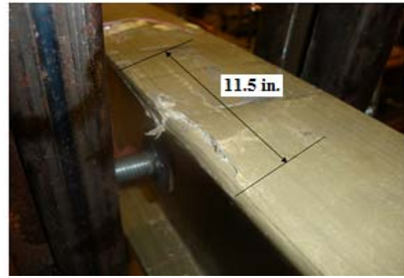
Fig. 4 : Top flange GFRP beam cracking in Experiment 1
