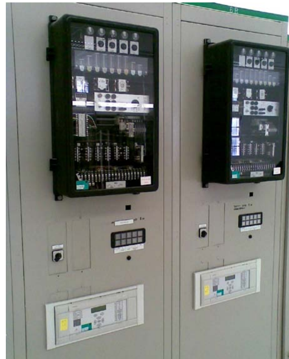
Figure 2 : Section of Distance Protection panel for critical 160 kV lines consisting of electromechanical relays type LZ31 (above) connected in-parallel with microprocessor-based protection MiCOM P437 (bottom)
