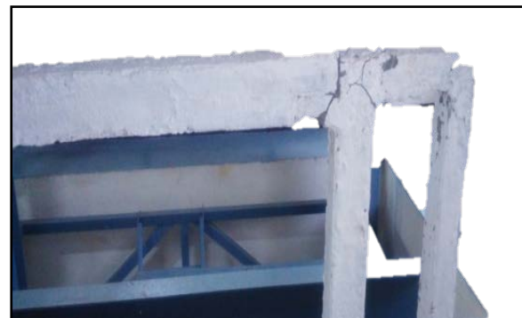
Figure 6b : Damage pattern for M3
