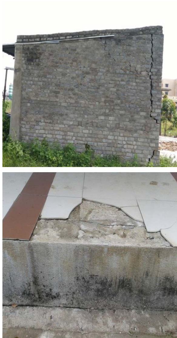
Figure 1 : Cracks, Swelling in Black cotton soil
