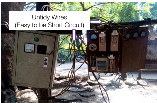
Fig. 13: Distribution Board of Mini-Grid
