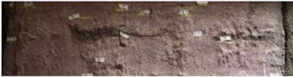
Figure 10: Interruption trace of concreting on a panel of diaphragm wall [7]
