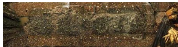
Figure 8: Difference of concrete inside and outside the reinforcement cage [7]
