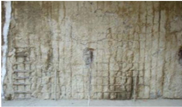
Figure 3: Panels with exposed rebars [9]
