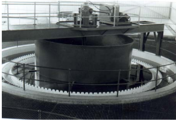
Figure 23: The Saulspoor waterworks – the HR clarifier, design capacity 10 \text{ ML.d}^{-1}
