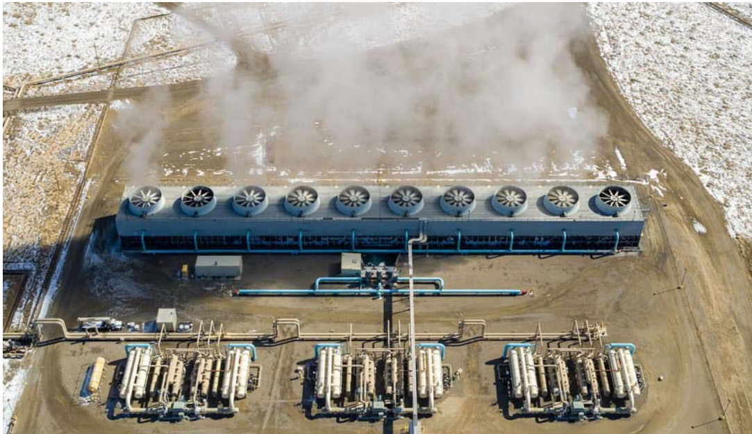
Fig. 4.5.1: Fervo Energy's 3.5-megawatt enhanced geothermal plant in Nevada. Credits to Google/Fervo Energy
