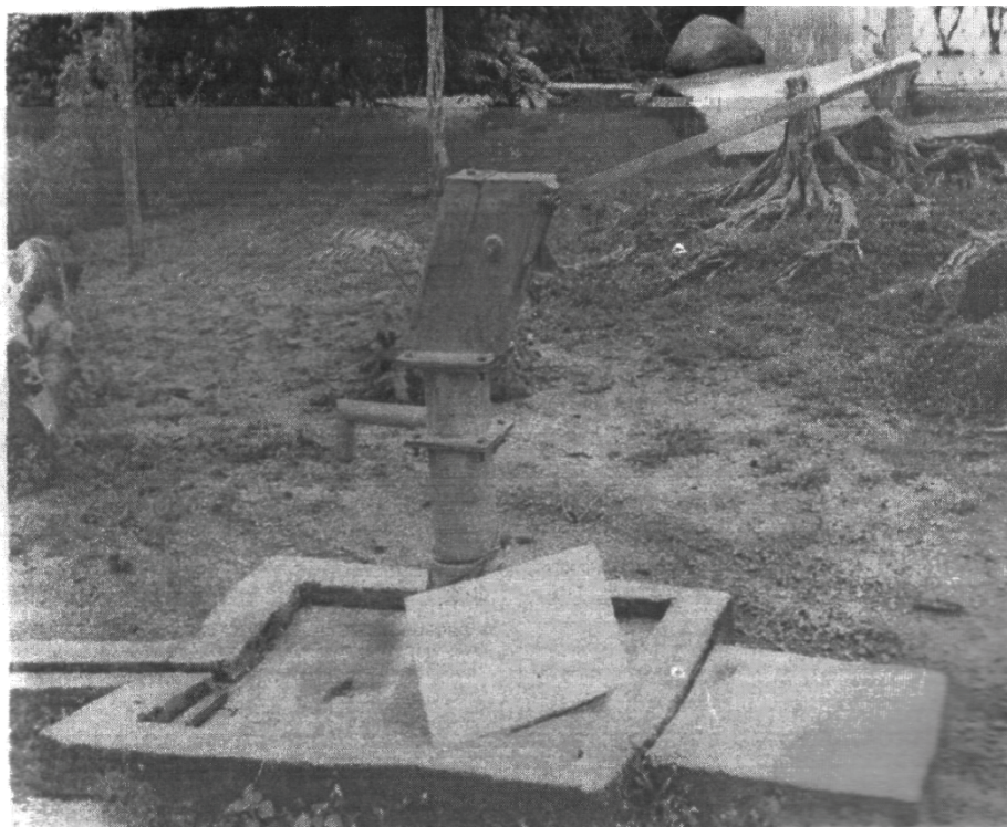
Plate 3 : Non-functioning hand pump water supply system at Iwere-ile.
