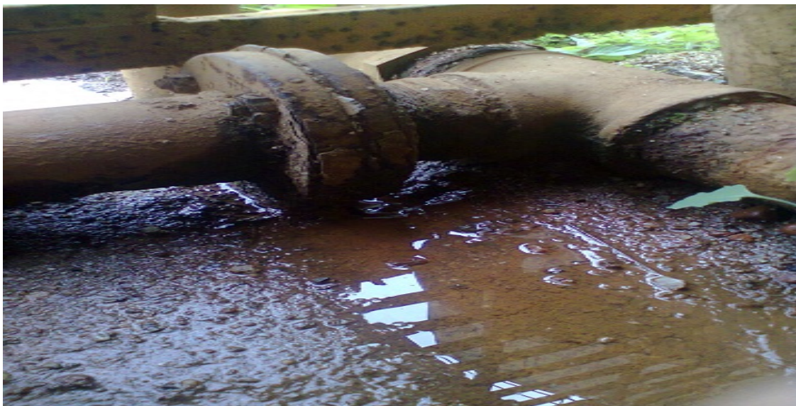
Plate 1 Leakage from the burst pipeline
