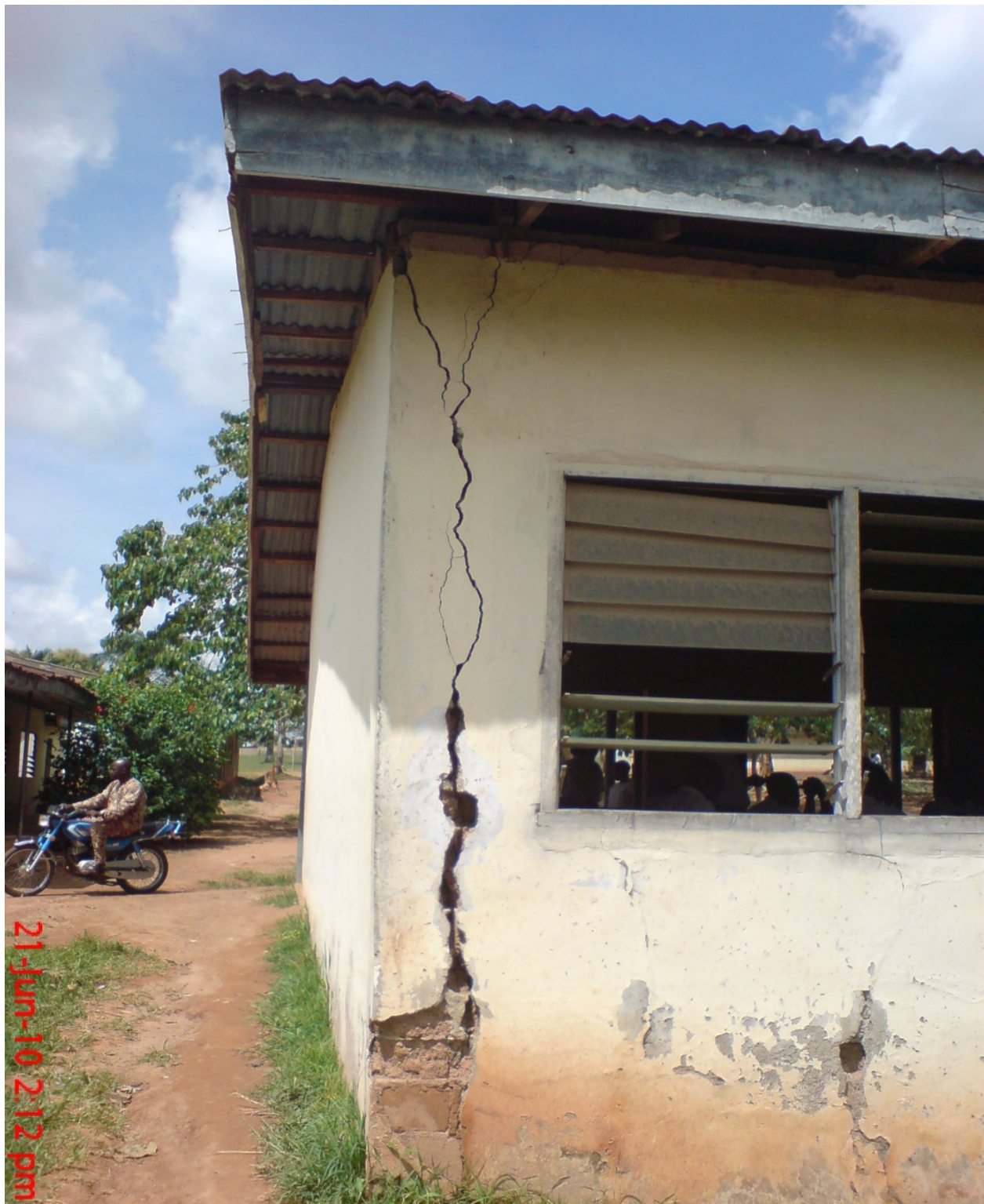
Figure 7 : Showing the Cracks in the Building Named Block 3 Located Along Traverse 4
