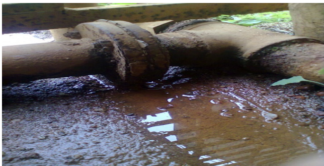
Plate 1 : Leakage from the Burst Pipeline
