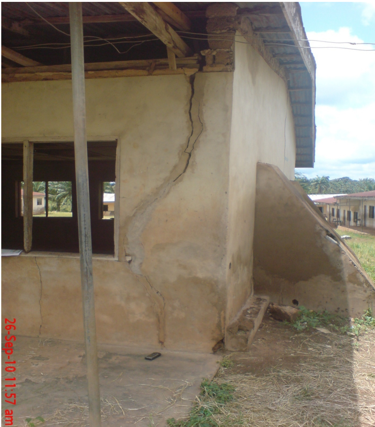
Figure 5 : Showing the Cracks in the Building Named Block 1 Located Along Traverse 3
