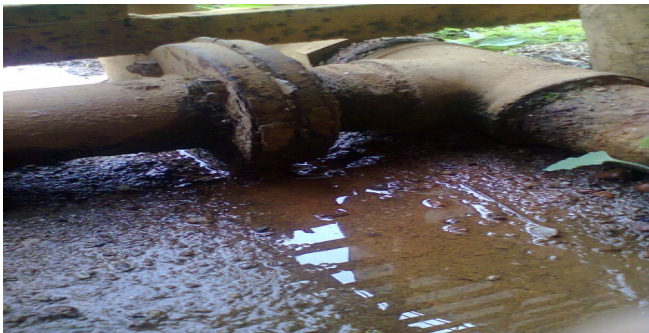
Plate 1 : Leakage from the Burst Pipeline
