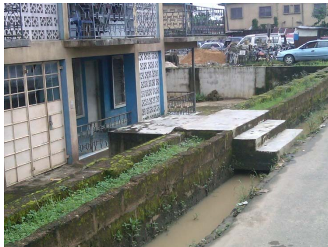
Plate 3: Sunken compound at Nsentip Street flood area
