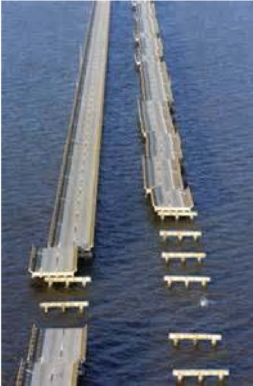
Fig. 5 : Interstate I-10 over Mobile Bay damaged by Hurricane Ivan in 2004(From FHWA-NHI-07-096).According to FHWA, the wave setup on top of the storm surge was the cause
