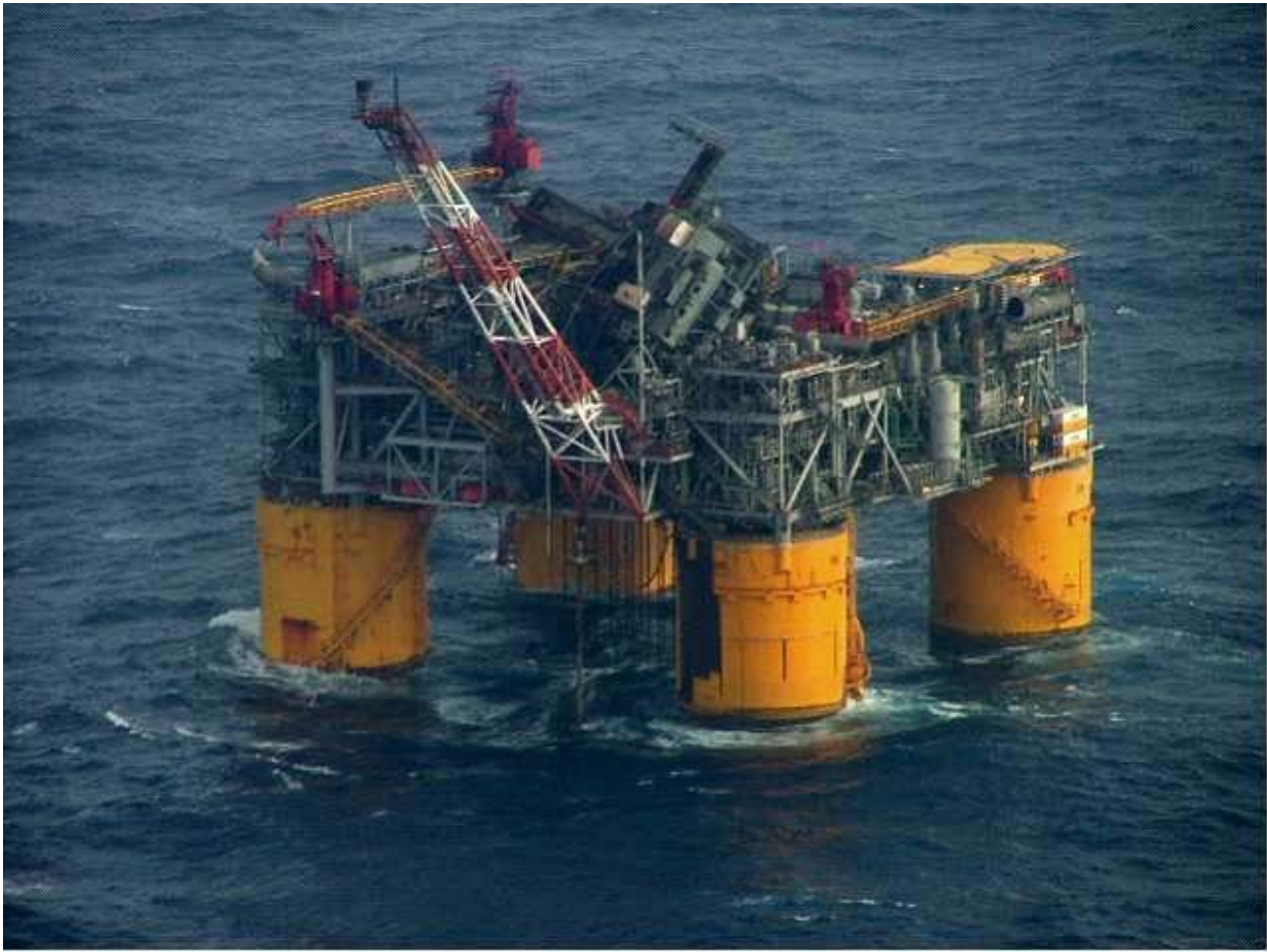
Fig .4 : Mars platform showing damage from Hurricane Katrina in2005( http://en.wikipedia.org/wiki/Mars_(oil_platform) ). According to Wang and Oey (2008), this billion-dollar platform was designed to withstand “140-mph winds and crashing waves up to 70ft high simultaneously”
