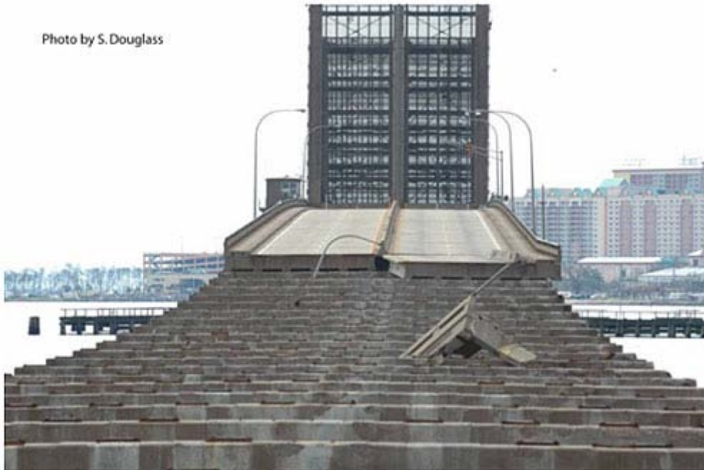
Fig. 6 : US 90 bridge over Biloxi Bay, Mississippi, was damaged by Katrina. Since the spans at higher elevations were not removed, the wave setup on top of the storm surge is more important than the wind loading (photo looking southwest from Ocean Springs 2/19/06, from FHWA-NHI-07-096)
